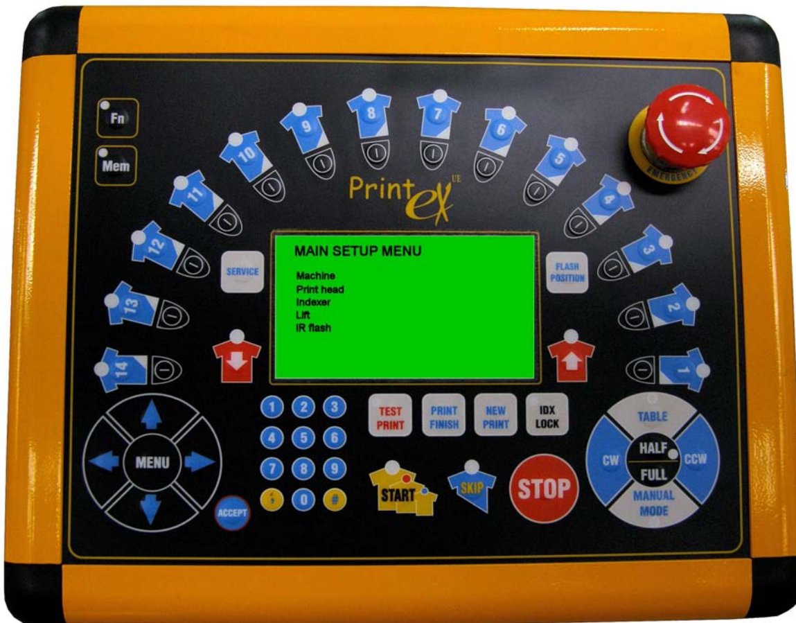
Fig. 21: MAIN CONTROL PANEL
